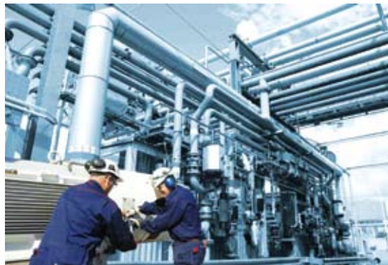
The IECEx Certified Persons Scheme will provide industry with a one-stop solution.
